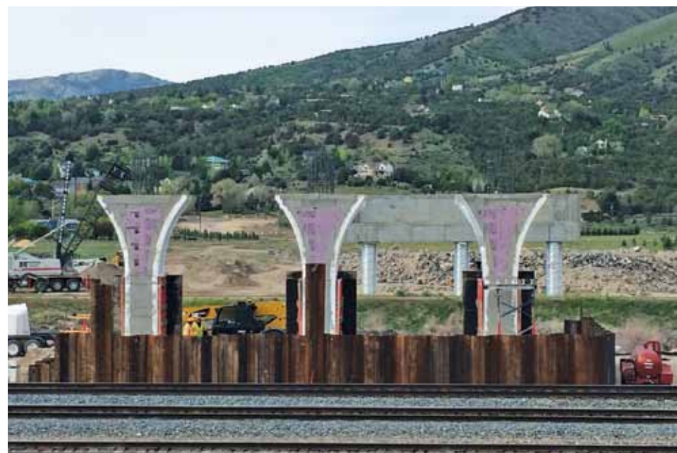
EPS Geofoam was effectively utilized on the Cheyenne South Valley Connector project in Pocatello, Idaho.
